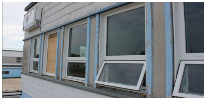
Replacement windows being installed at Weeneebayko General Hospital with some windows locations eliminated - awaiting filler panel installation, insulation, flashing, trim, and caulking.
