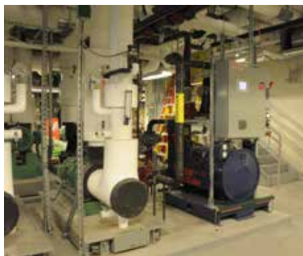
▲ The fuel gas booster located in the penthouse mechanical room is used to raise the pressure of the fuel gas to the operating level of the combined heat and power (co-generation) plant located on the roof. Photo courtesy Kent Waddington Photography.
