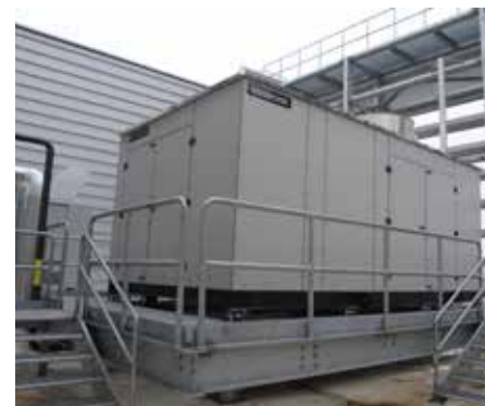
▲ The roof-mounted 250 kilowatt gas-fired co-generation plant produces both heat and power, adding to Spaulding's ability to be energy-efficient and remain operational during times of natural calamity. Photo courtesy Kent Waddington Photography.
